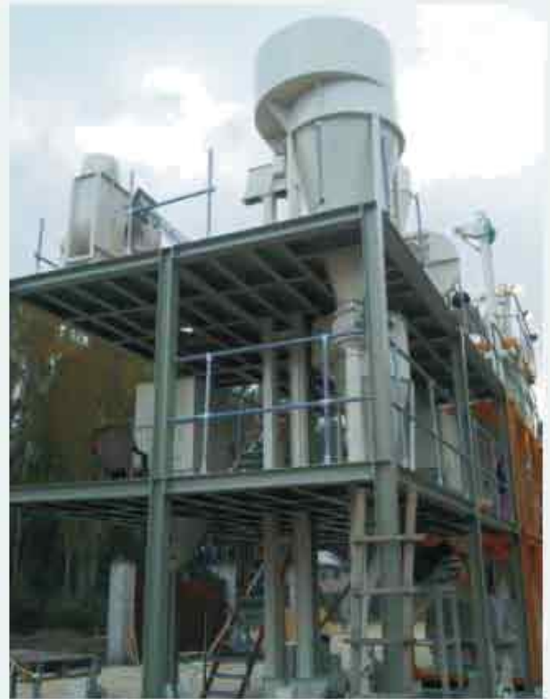
Installation of Trout Feed Mill plant, Imported by STC for Directorate of Fisheries, Govt. of Jammu & Kashmir.
